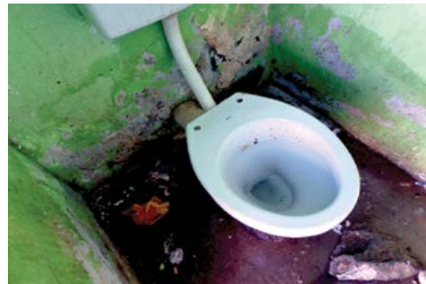
A shared flushing toilet in Havana shown by a resident as an example of the unhygienic conditions in the settlement
